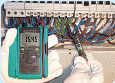
Measuring current in a Switchboard
